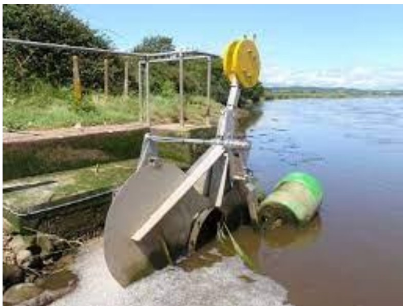
Plate 5 Self regulating tide gate at Seaton in Devon (Figure 3.6 in https://assets.publishing.service.gov.uk/media/6033a8f5e90e076607c1bf0e/Self-regulating_tide-gate_a_new_design_for_habitat_creation_technical_report.pdf )
